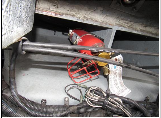
FIRE SUPPRESSION SYSTEM
