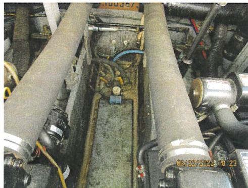
ENGINE ROOM CENTER & BILGE
