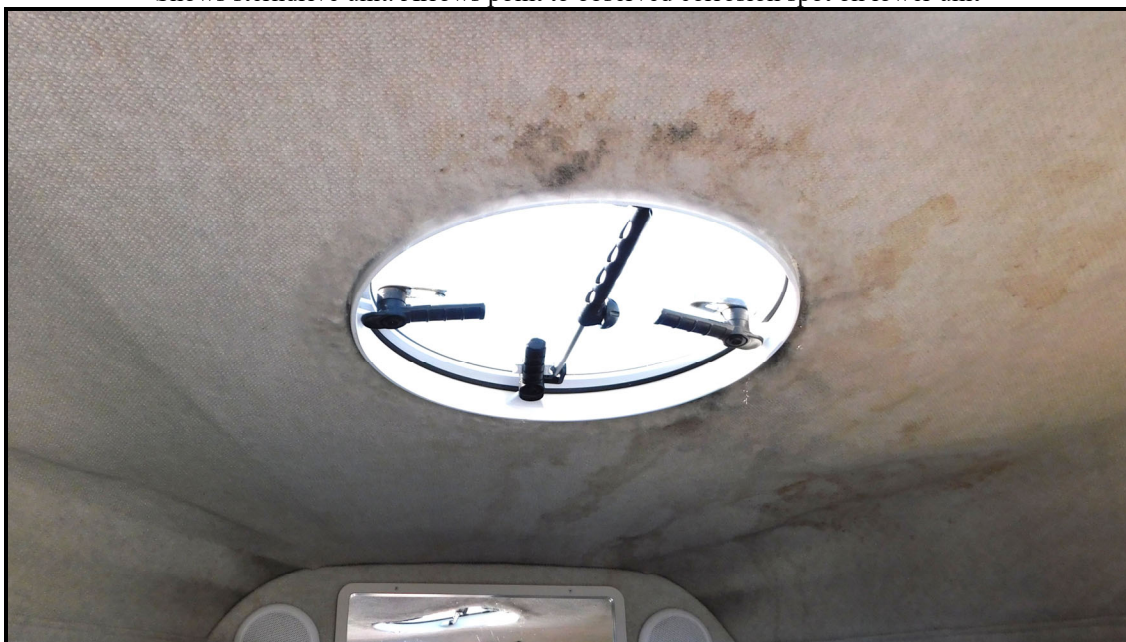
Shows observed water stain in cabin headliner from prior water intrusion
