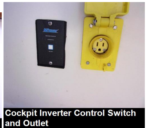
AC Power Distribution Panel
