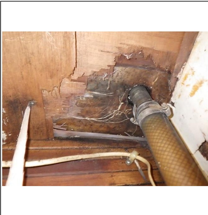
Deteriorated deck structure as sighted from the cabin.
