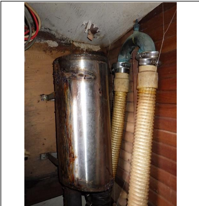
Stainless steel muffler for engine has crevice corrosion, and is leaking.
