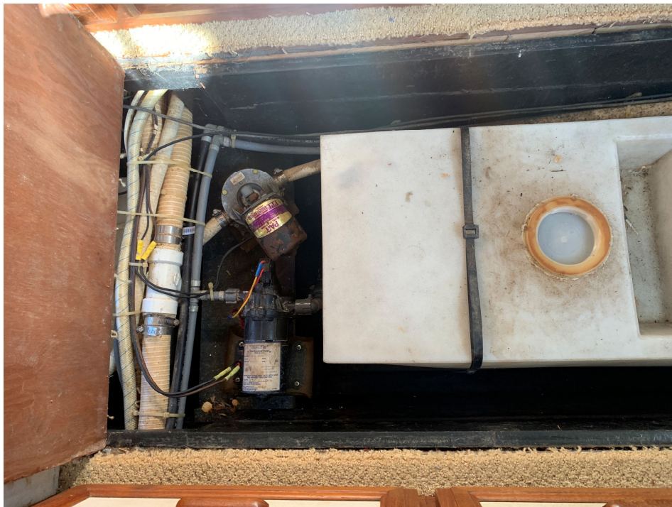
View of plumbing in cabin bilge compartment
