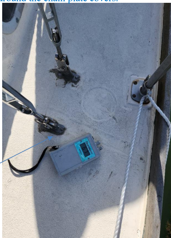
Pic #7 There are elevated moisture levels and delamination on the starboard side deck in a 4 foot area midship near the chain plates with minor gelcoat cracks around the chain plate covers.
