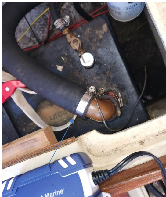
Pic #5 The fuel tank fill hose is only single clamped at the tank and it is a federal requirement that fuel fill hoses are double clamped. Add clamps as needed.
