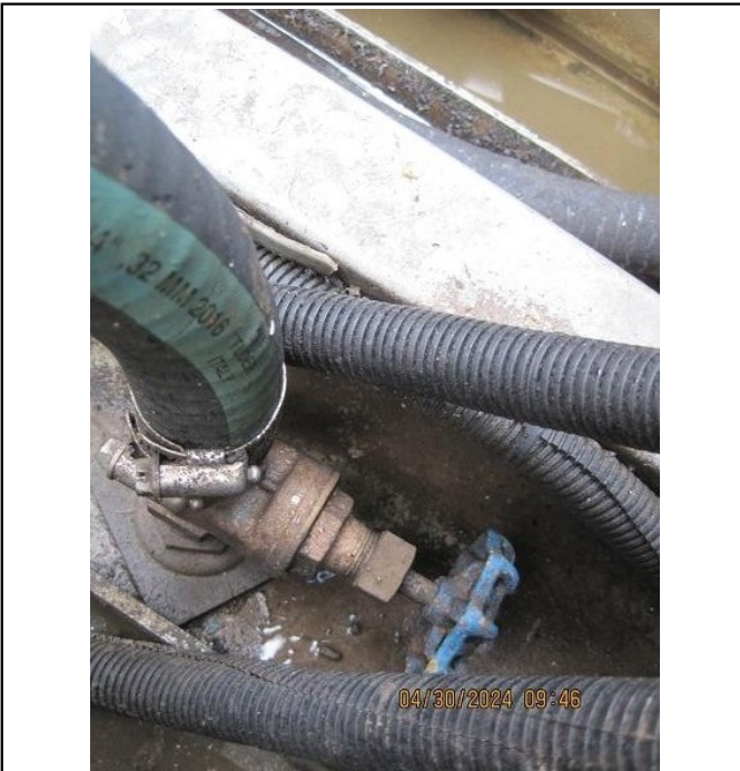
Raw water engine intake and gate valve.
