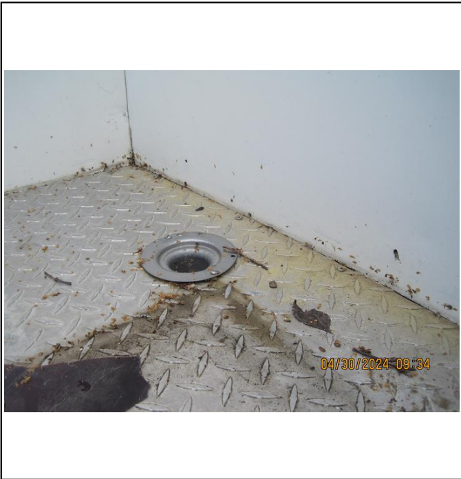
Aft cockpit starboard drain.
