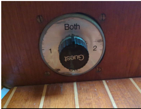
GUEST battery switch
