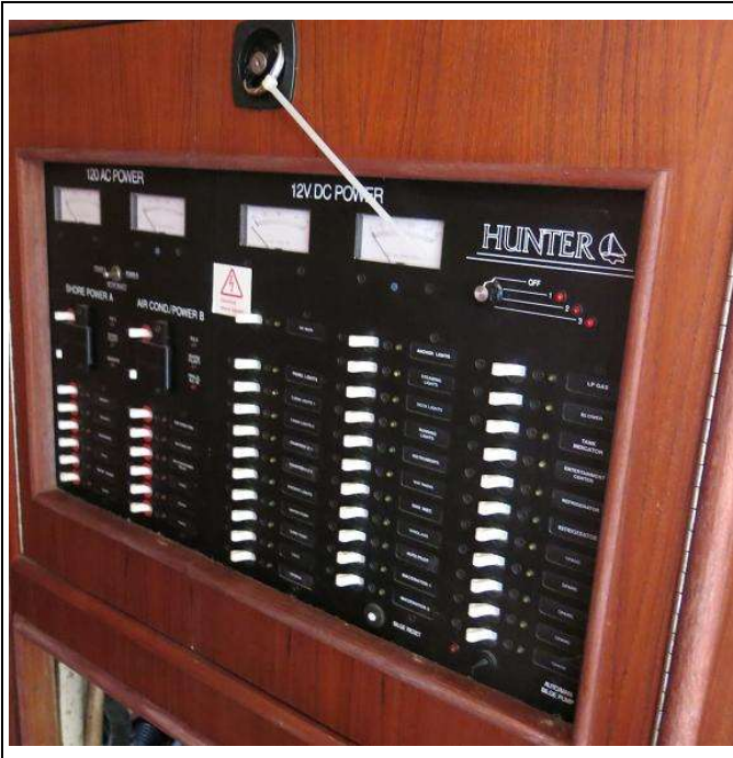
Main Electric Panel
